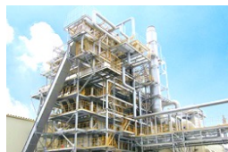
Biomass power plants
