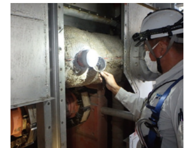
An equipment inspection
