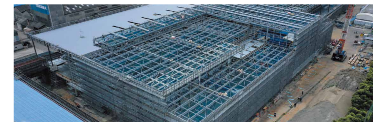
(Photograph of construction progress at the new Harima Factory) Date: June 16, 2022 Scheduled completion: December 2022 Capital investment: Approx. JPY 13 billion
