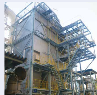
Waste heat boiler
