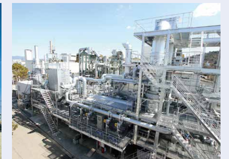
Sewage sludge-fueled power plant
