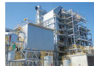
Biomass power generation boiler
