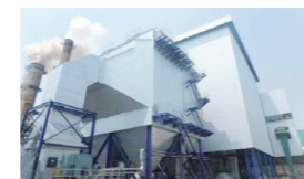
Bagasse-Fired Boiler Plant (Thailand)
