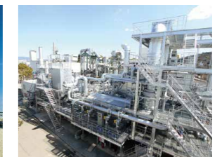
Sewage sludge-fueled power plant system
