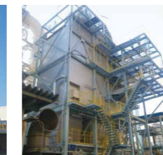
Waste heat boiler
