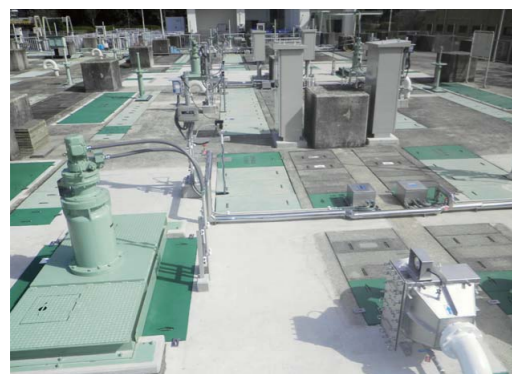
Installation example (Higashiujii Sewage Treatment Plant, Uji City)
