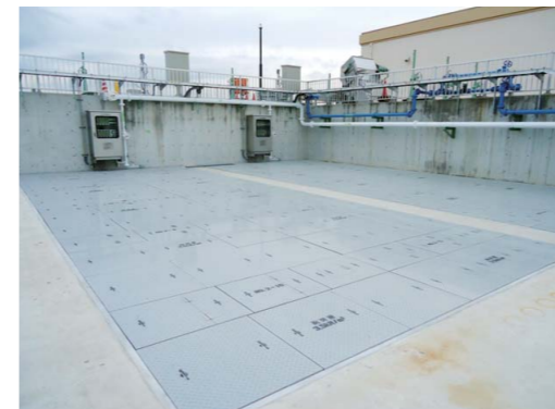
Installation example (Edagawa Sewage Treatment Plant, Nishinomiya City)
