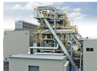
Biomass power plant
