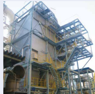
Waste heat boiler
