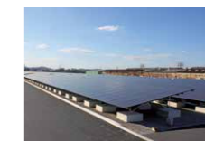
(11) Takuma Solar Power Plant
