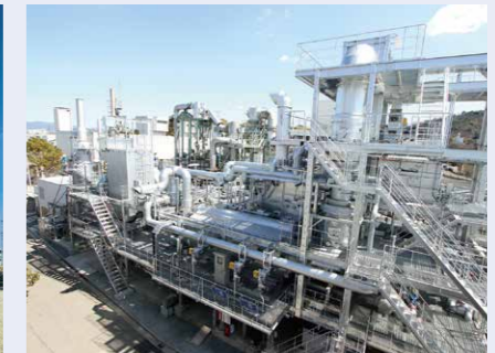
Sewage sludge-fueled power plant
