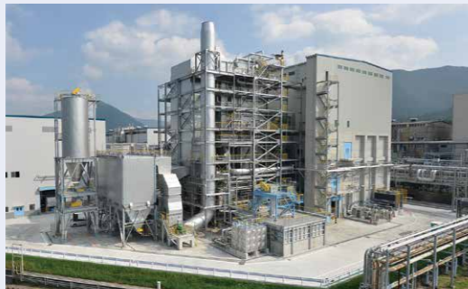
Biomass power generation boiler
