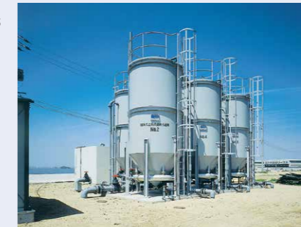
Upflow moving-bed sand filtration system
