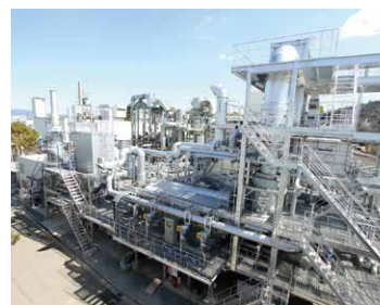
Sewage sludge-fueled power plant
