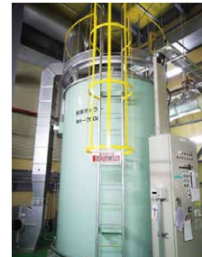
Heat Medium Oil Boilers Thermoheater
