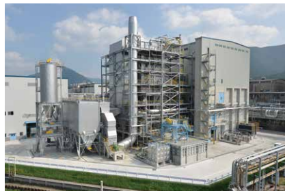
Biomass power generation boiler
