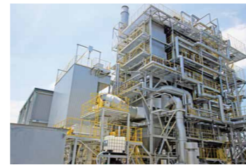
Biomass Power Plant
