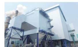
Bagasse-Fired Boiler Plant (Thailand)
