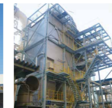
Waste heat boiler
