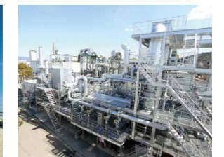
Sewage sludge-fueled power plant system
