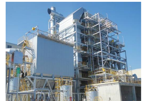
Biomass power plants
