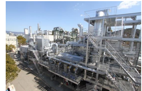
Sewage sludge power generation system
