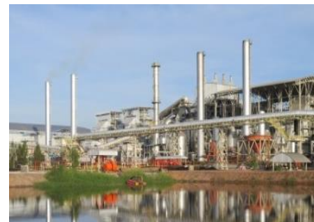
Bagasse Fired Boiler Plant (Thailand)
