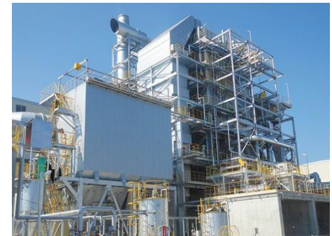
Biomass power plants
