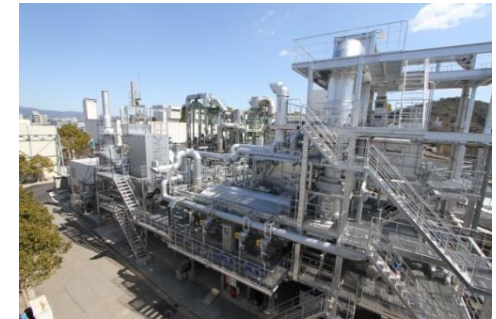
Sewage sludge power generation system
