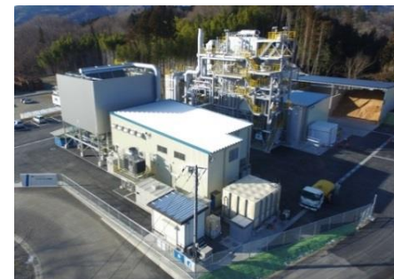
Biomass Power Plant
