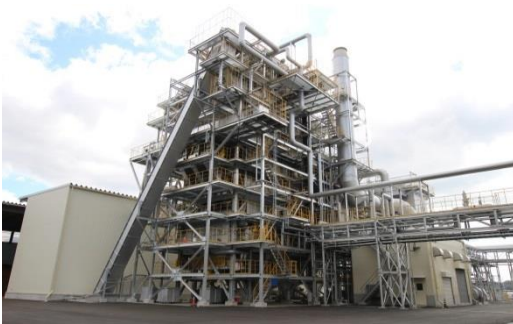
Biomass power plant
