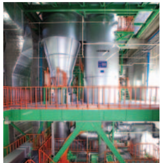
Circulating Fluidized-Bed Incinerator for Sewage Sludge
