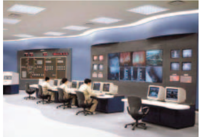
Control room for waste incineration plant
