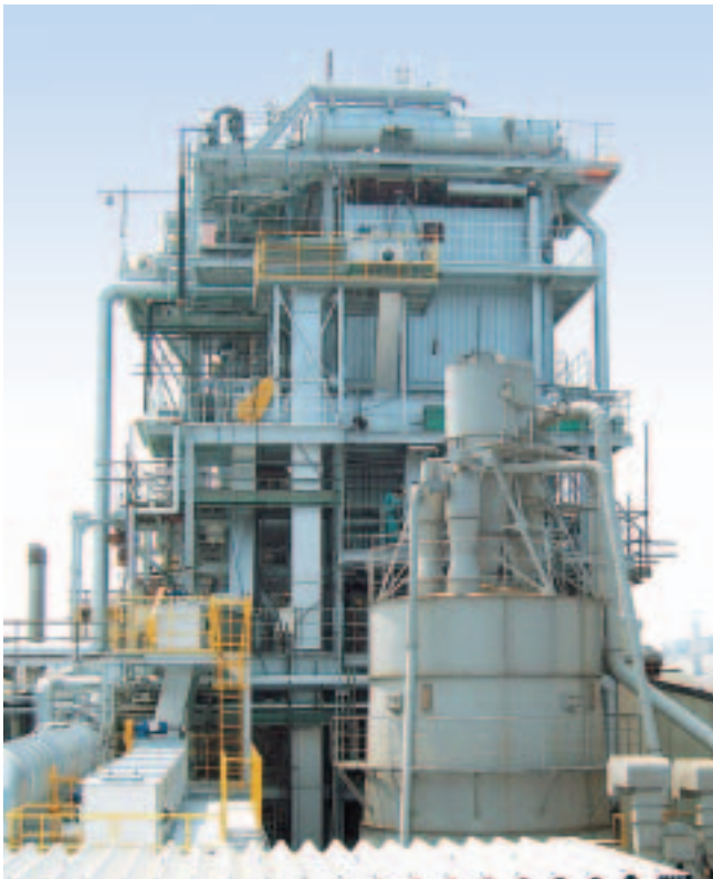
Biomass Boiler for Power Generation
