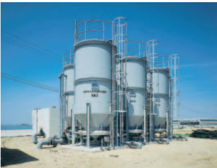
Continuous up-flow sand filter
