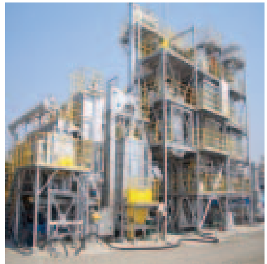
Demonstration plant of sewage sludge gasification and power generation
