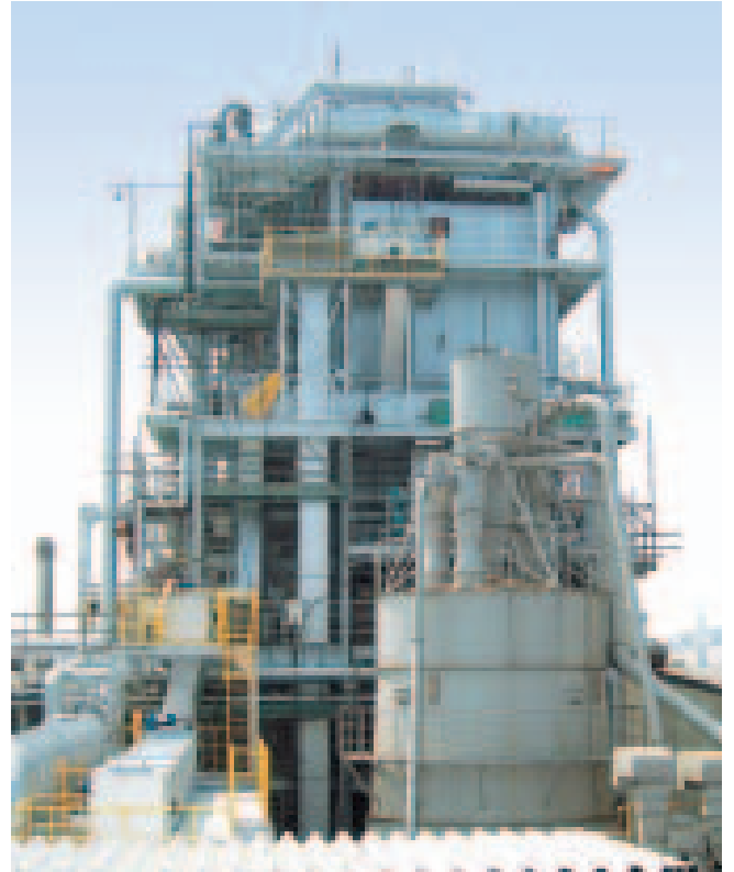
Biomass Boiler for Power Generation
