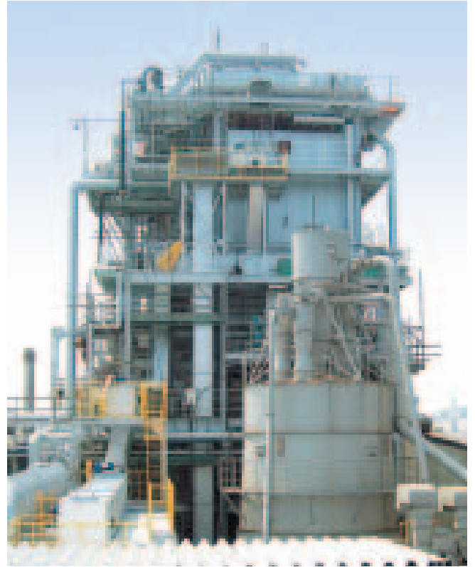
Biomass Boiler for Power Generation
