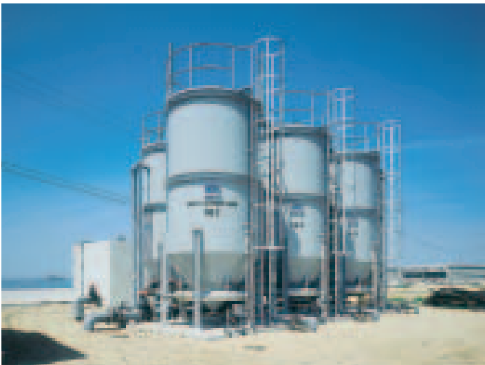
Continuous up-flow sand filter
