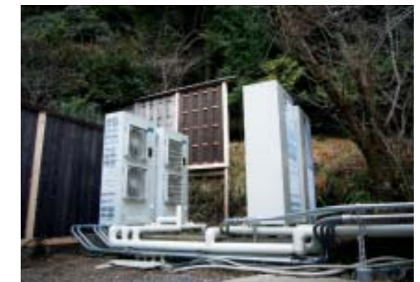
Accommodation with hot spring in Kyoto City (Delivered 4 units of heat pump water heater)
