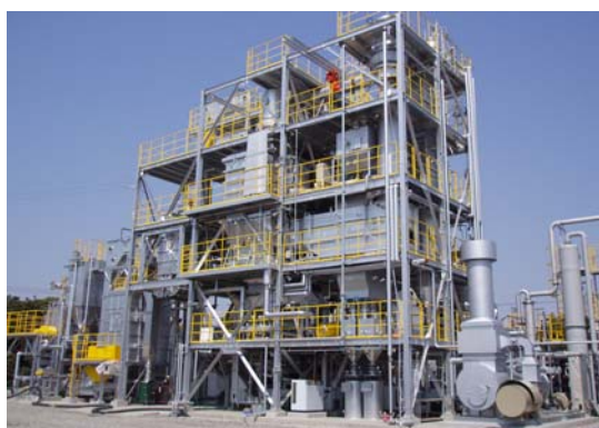
Sewage Sludge Gasification and Power Generation Demonstration Plant
